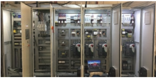
Control Panel During Commissioning
