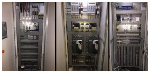
Control Panel Sections
