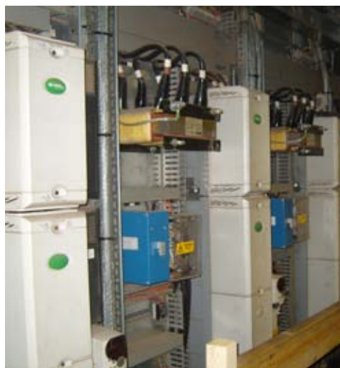
Unidrive SP Drives in-situ
