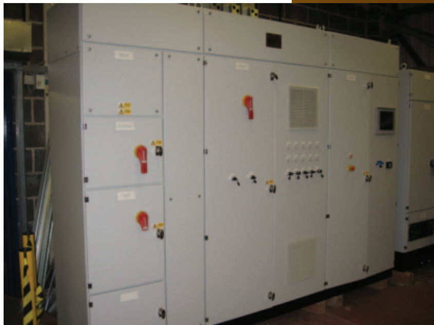
Motor Control Centre
